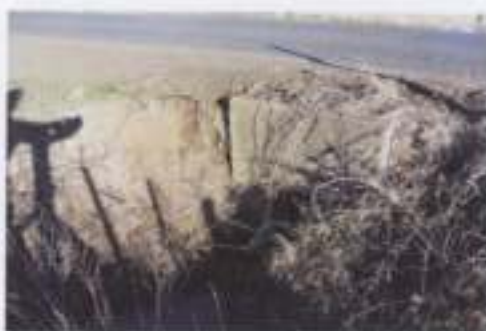
Fig. 2 Vegetation killed on steep embankments around culvert intakes leads to erosion of soil and gravel, pollution of watercourses by suspended particles and siltation of our estuaries.
