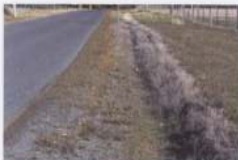
Fig.3 Herbicide applied once, from the paved edge across the table drain. Short lifecycle weeds are starting to dominate on the gravel shoulders. More frequent spraying is required to keep weeds from seeding into the bare area as well as into neighbouring properties.
